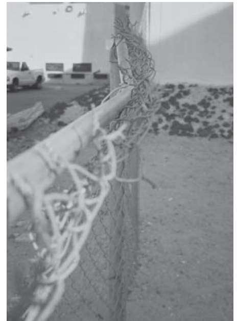
Broken Fence Fatimah Martin, Grade 11
